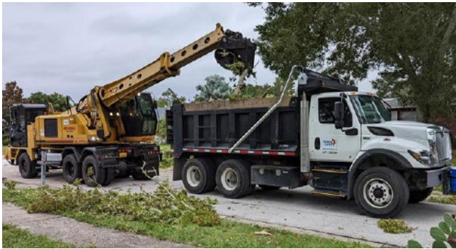
A total of 16 Pinellas County Public Works crews hit the road early Thursday, September 29 for the first push after Hurricane Ian. Crews were assessing damage, clearing minor debris and reporting priority work requests.
